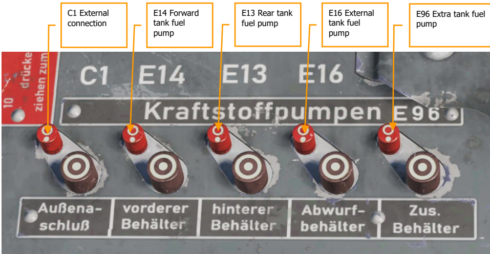
Figure 77: Fuel system circuit breaker
