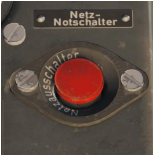
Figure 70: Electrical system killswitch
